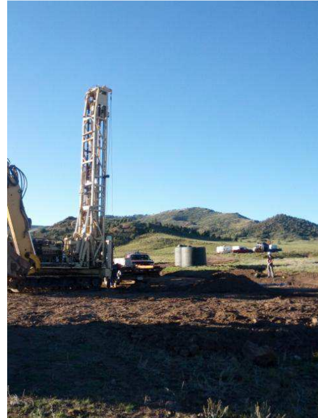
Installation of a water monitoring well at the Hansen Deposit during October 2013
