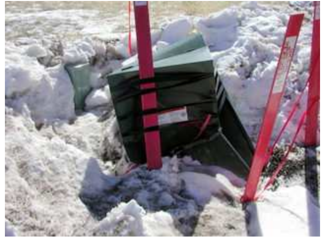
Damaged box near the intersection of South T-Bar Trail & Sphar Court.
